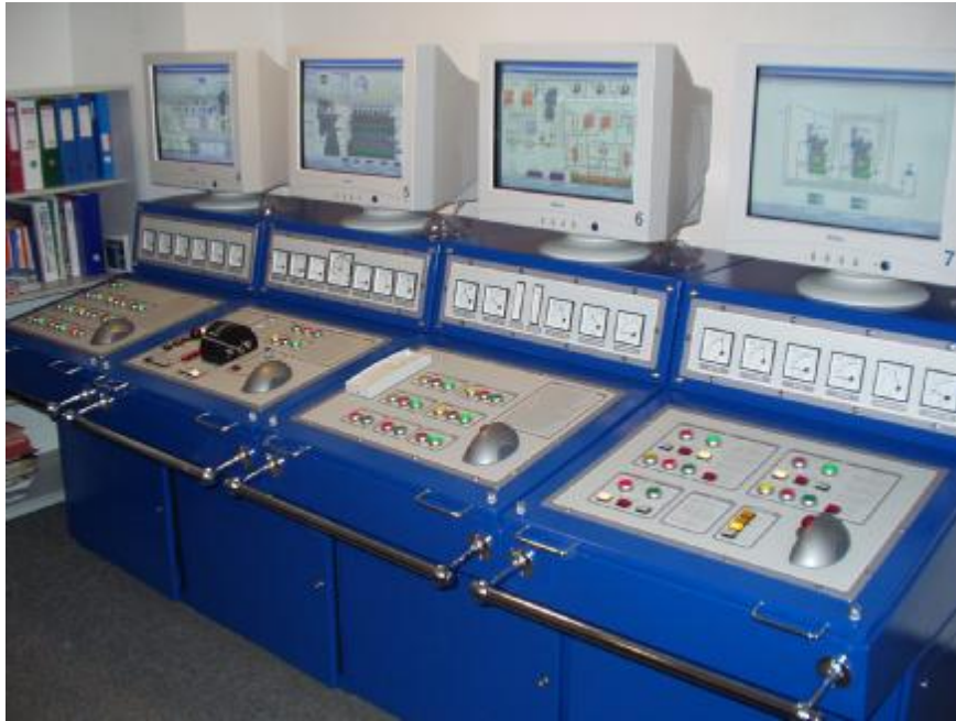
Fig. 1 The set of control consoles.
